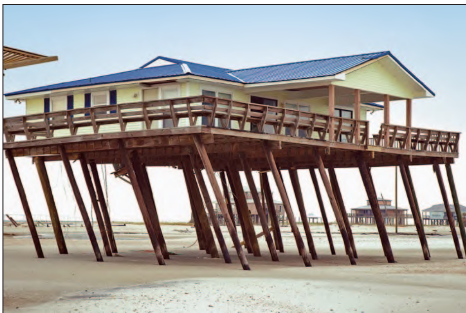
Figure 10-2. Near collapse due to insufficient pile embedment, Hurricane Katrina (Dauphin Island, AL, 2005)
