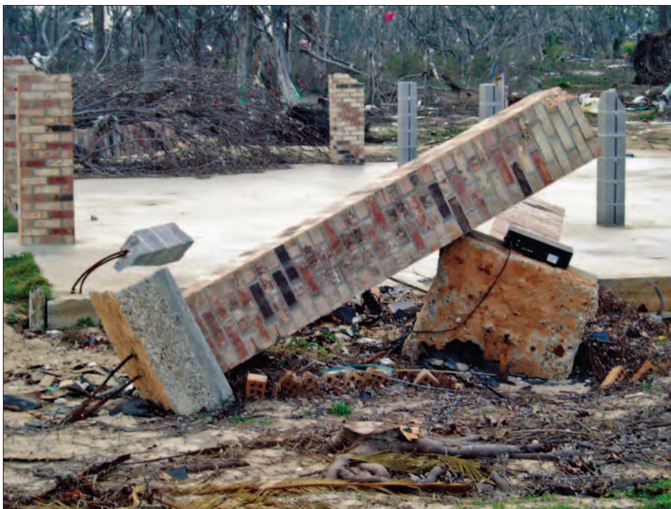
Figure 10-17. Performance comparison of pier foundations: piers on discrete footings (foreground) failed by rotating and overturning while piers on more substantial footings (in this case a concrete mat) survived Hurricane Katrina (Pass Christian, MS, 2005)
